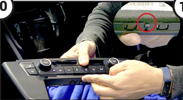
Relocate the climate control button panel into the new double DIN fascia panel, ensuring that the middle clip is lined up for a perfect fit
